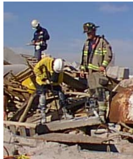
Figure 1: A firefighter (with white hat) views the portable screen of a search cam which is probing below a concrete slab.
